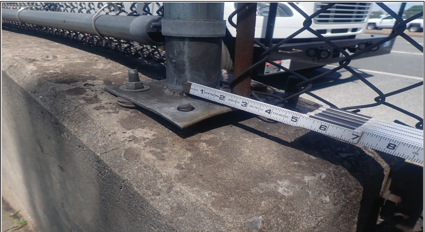
22 SOUTH METAL RAIL FENCE MISSING PARAPET CONNECTION AT THE EAST END
