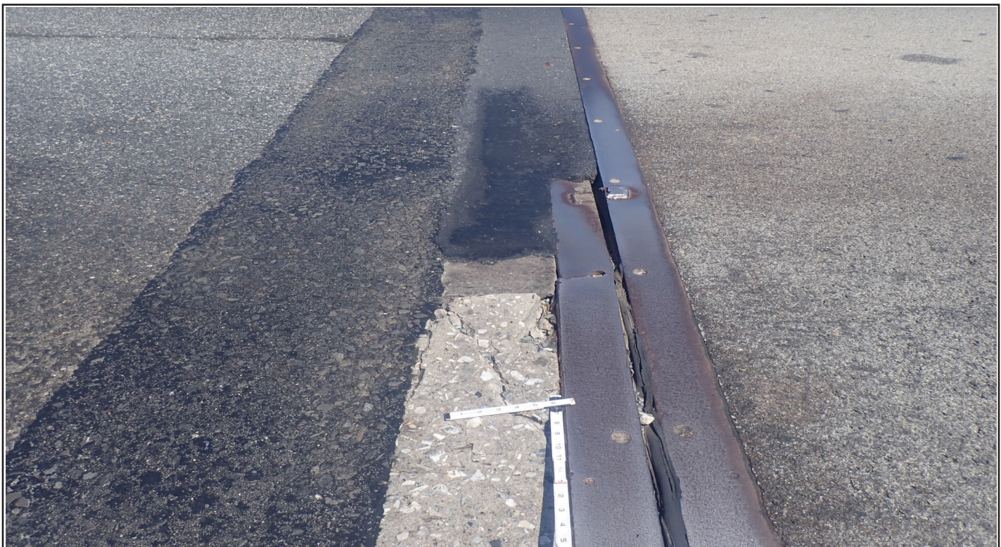
16 WEST ABUTMENT BACKWALL TOP SIDE DEEP SPALLS AND ASPHALT PATCHES IN EASTBOUND LANE
