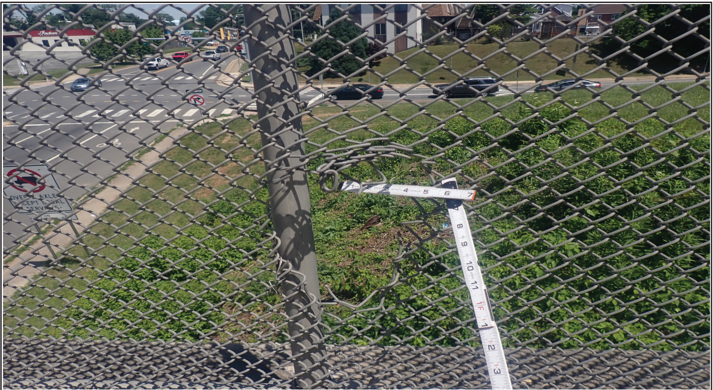
20 NORTH METAL RAIL FENCE HOLE OVER THE EAST ABUTMENT
