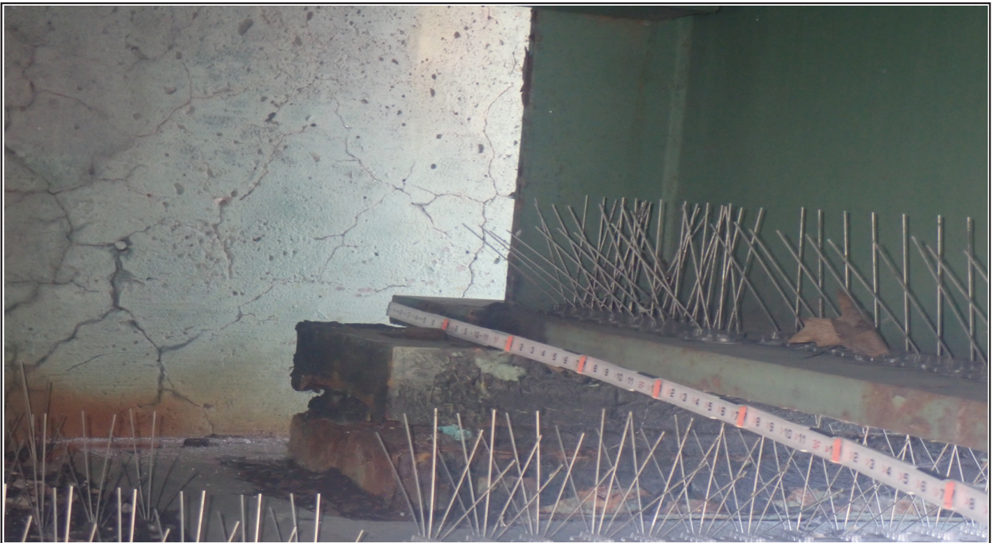
12 WEST ABUTMENT MOVEABLE BEARING 1 MISSING CONNECTION
