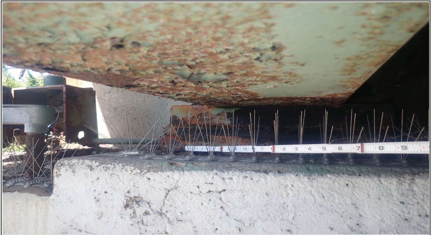
15 WEST ABUTMENT MOVEABLE BEARING 15 CORROSION w/LOSS OF SECTION
