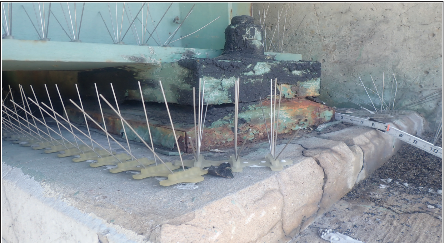
10 EAST ABUTMENT FIXED BEARING 15 CORROSION w/LOSS OF SECTION
