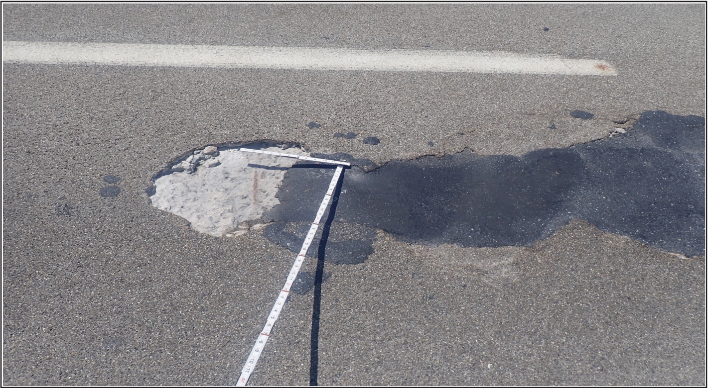
21 DECK EXP BAR w/ASPHALT PATCH IN WESTBOUND LANE
