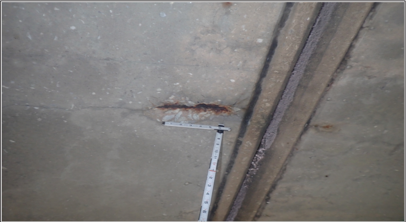
13 SOFFIT EXP BAR w/LOSS OF SECTION IN BAY 7 OVER WEST SIDEWALK
