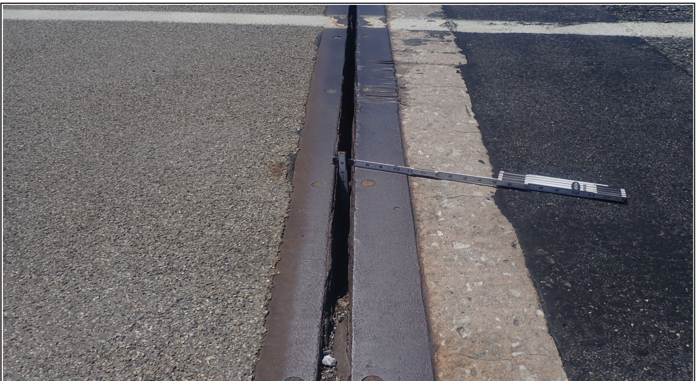
18 WEST COMPRESSION JOINT MISSING IN THE WESTBOUND LANE
