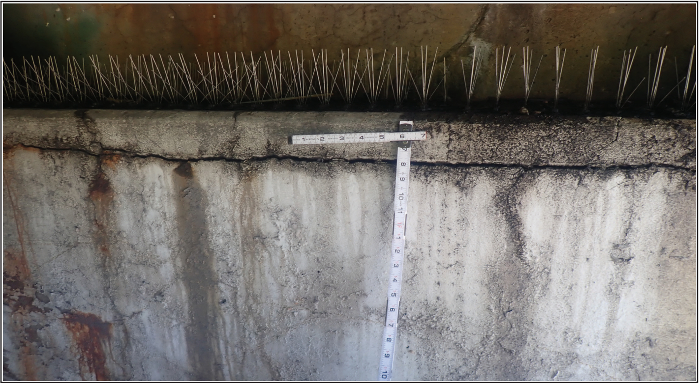
7 EAST ABUTMENT WIDE HORIZONTAL CRACK UNDER BAY 14
