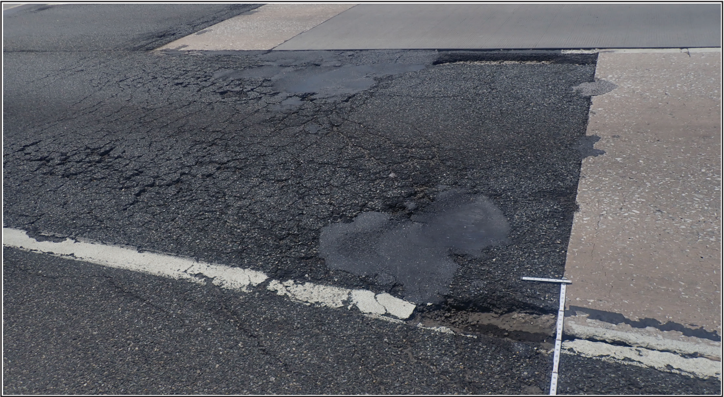
19 NORTHWEST ASPHALT APPROACH SLAB DEEP SPALLS w/DETERIORATING ASPHALT
