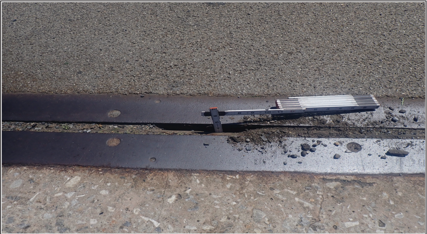
17 WEST COMPRESSION JOINT FULLY DEBONDED IN THE EASTBOUND LANES
