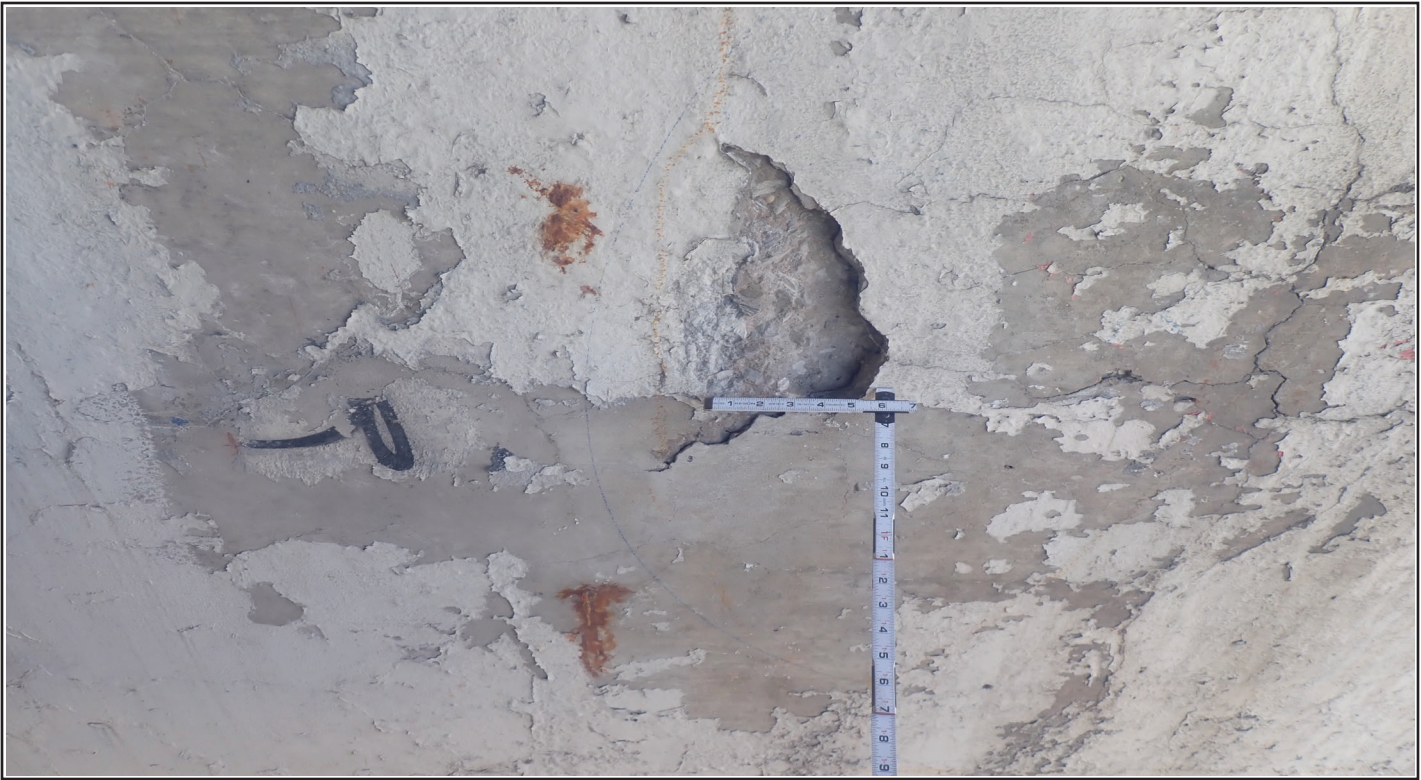
11 EAST ABUTMENT BREASTWALL DEEP SPALL UNDER GIRDER 14
