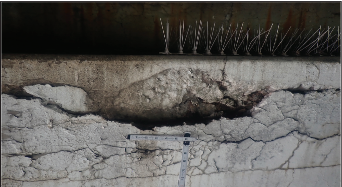
14 WEST ABUTMENT EXP BAR w/LOSS OF SECTION UNDER BAY 10
